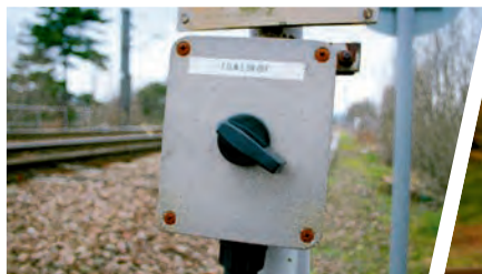
Example of a TOWS switch
