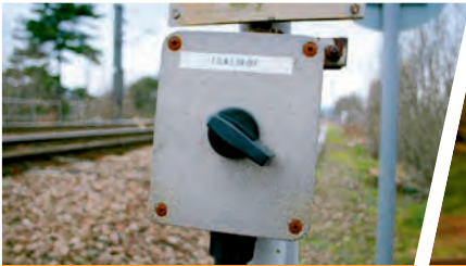
Example of a TOWS switch
